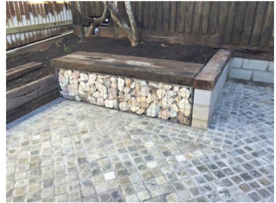
A garden seat using gabions and tuff rock supplied by Caged Rock.
